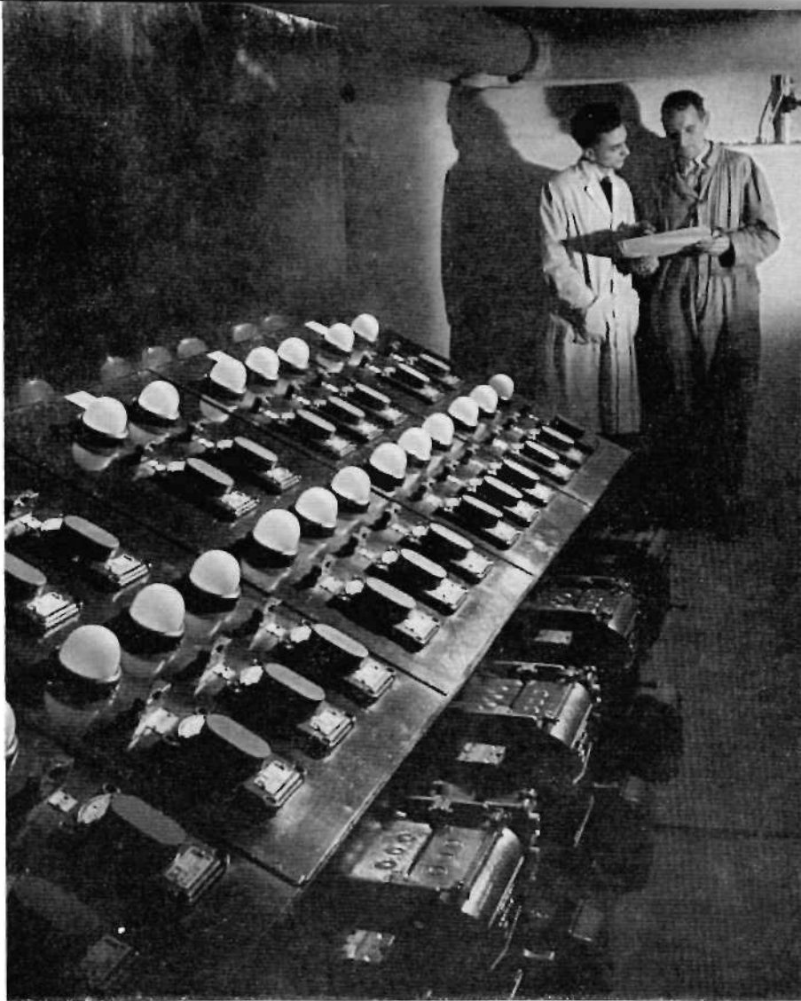
Control panel of air-conditioning plant at an Ilford factory.
